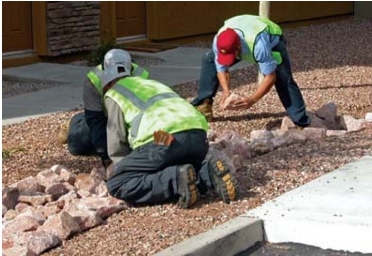
After this community was built, several areas drained water and began to wash away the decomposed granite. These areas are being dug out to create a channel and will be filled with Rip Rap to alleviate erosion and increase the aesthetic appeal.
